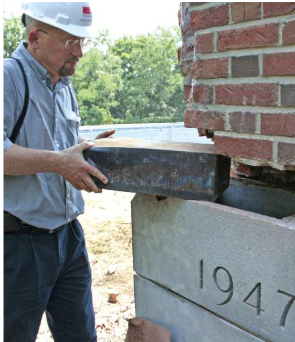
Construction Project Manager Kenneth Grizzell removes a time capsule from the cornerstone of Smith Hall.
