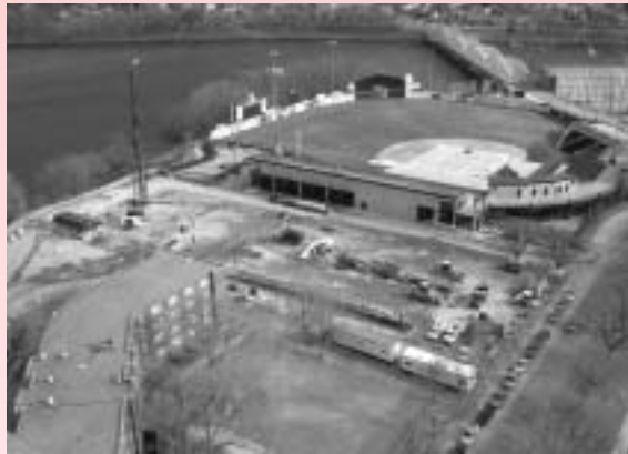
▲ The view from the roof of Fox Hall shows construction progress on the UML East parking garage.
